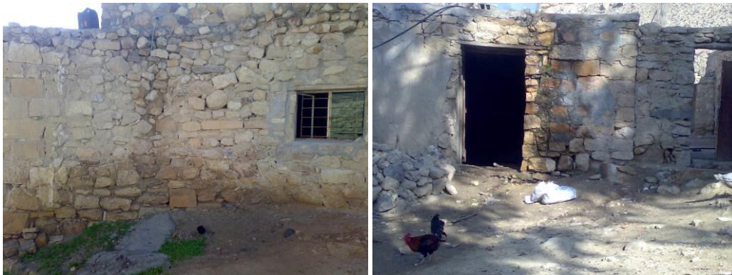
Fig. 14: The falling water affects the base of houses and walls cover.
