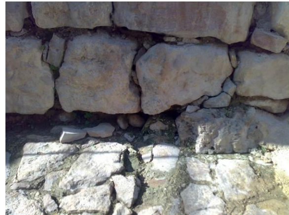
Fig. 16: The settlement of base
