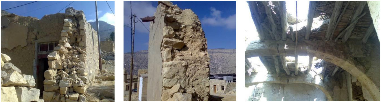
Fig. 5: After the ceiling fell, the rain washed off the mud plaster then deterioration started.
