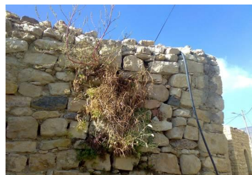
Fig. 4: Vegetative growth traps moisture breaking the walls cohesive bonds
